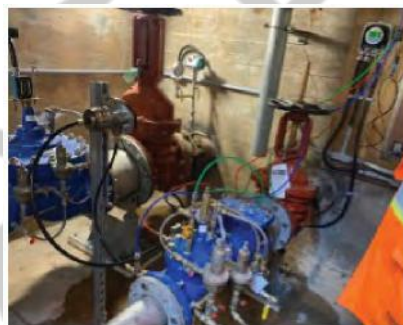
ADVANCED PRESSURE MANAGEMENT SYSTEM INSTALLED ON A PRV IN NORTH AMERICA
